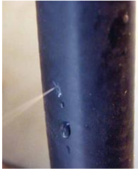
Example of a Fluid Jet Failure
